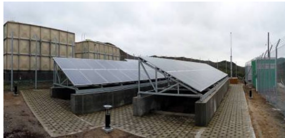
PV Panels installed at Dawn Island
